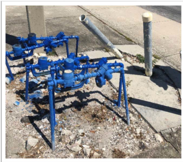
Above Ground Water Meters
