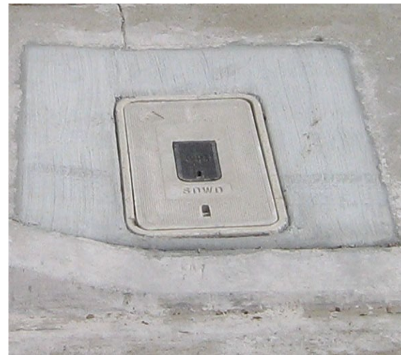
Underground Water Meters
